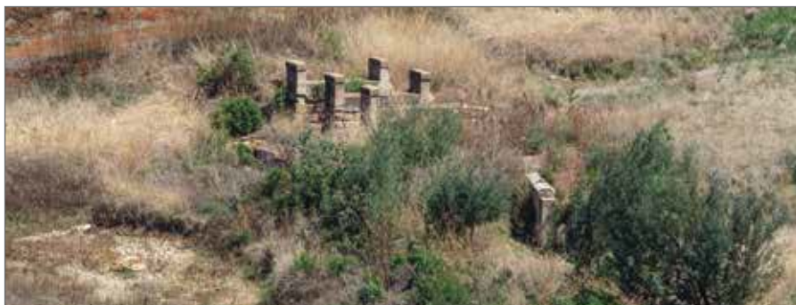
Figure 7: The remains of the two horseshoe bridges at Boscobello in September 2015 – the first in the background and the single remaining wall of the second in the foreground. During SA War 2, the three piers of the first bridge were damaged, the two end girders were dropped and the middle two girders cut
