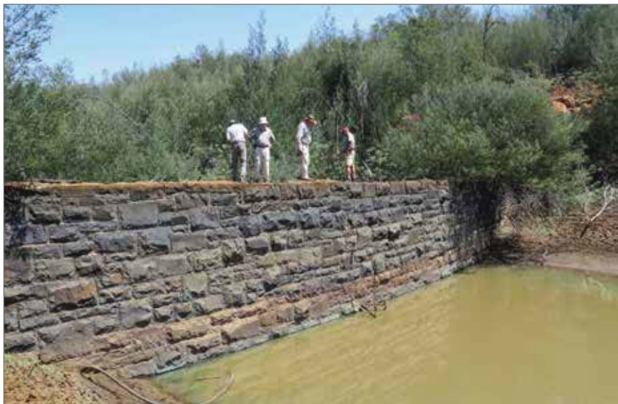
Figure 6: The BERRT 2015 group inspects a small dam at the end of the second reverse, built in fine stone masonry; it is not clear whether this dam was built during the first or second alignments
