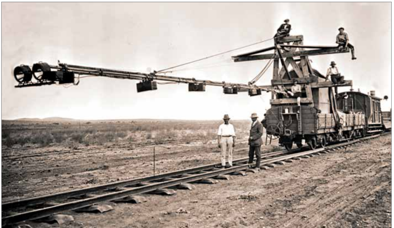
Figure 11: The lighting truck at the front, with the covered truck behind (Transnet Heritage Library photograph 18559)
