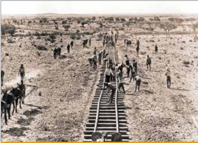
Figure 6: Different phases of tracklaying immediately ahead of the railhead (Transnet Heritage Library photograph 18565)
