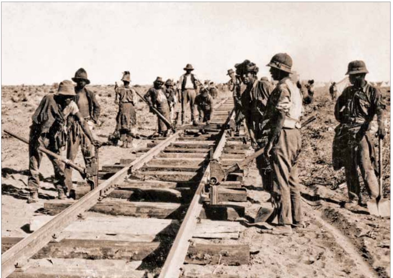
Figure 10: As soon as the rails were fished and fixed to the sleepers, "muck ballast" was shovelled up to the underside of the rails (Transnet Heritage Library photograph 18636)
